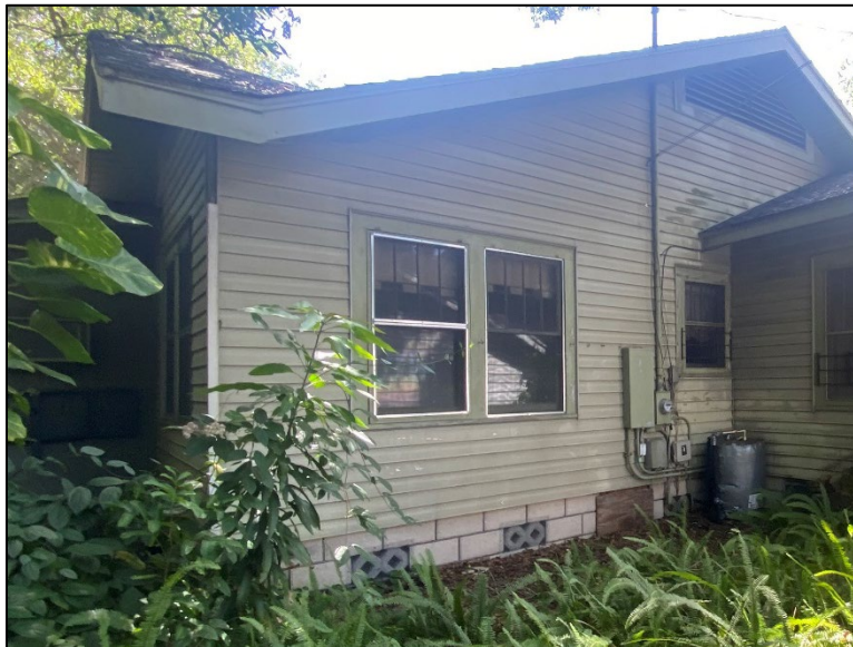
Figure 6: Historic (likely original) four-over-one wood double-hung sash windows found in a paired arrangement on the north elevation of the residence
